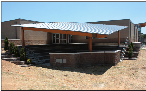
Construction on the Amphitheatre began in early spring. The new facility will seat 150 and will be used by the College for special events, as well as by the community.
